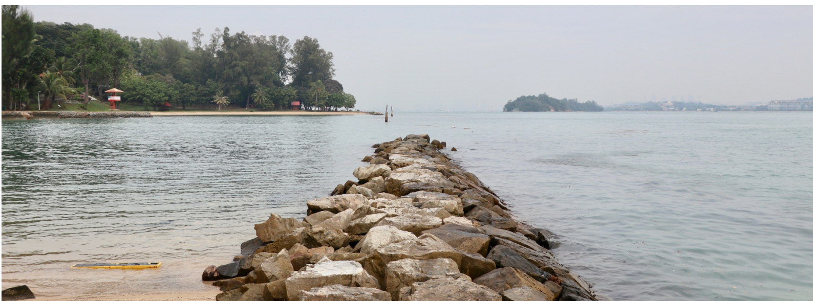
Figure 34 Seawall and breakwater constructed on SJI as a result of land reclamation and shoreline protection works on the island. Photo by Rachel Oh.
